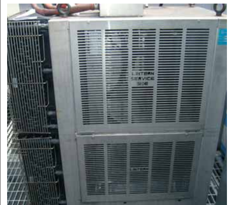
Lintern AC system with SRC coils attached
