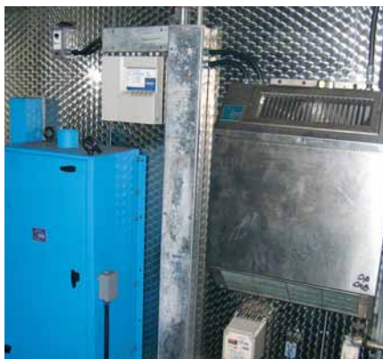
Lintern AC system inside a plant control centre
